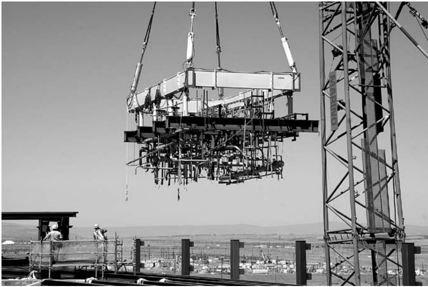
◀ A crane lifts a 19-ton piping module into the WTP's pre-treatment facility.
