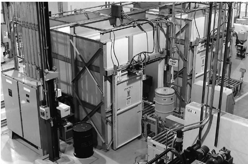
◀ An analytical cell inside the Waste Receiving and Processing Facility
