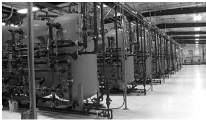
▲ Inside the 100-HX groundwater treatment facility.
