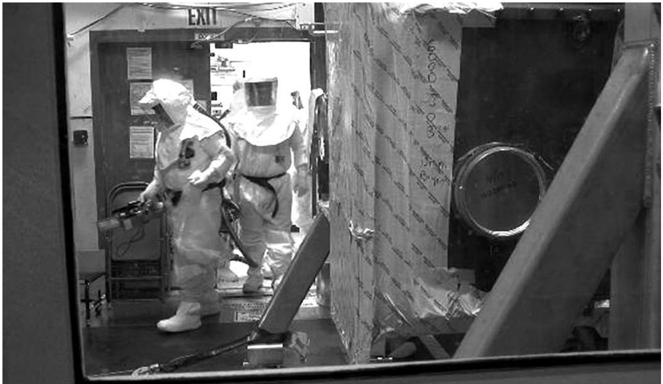
Workers in the Plutonium Finishing Plant. ▼
