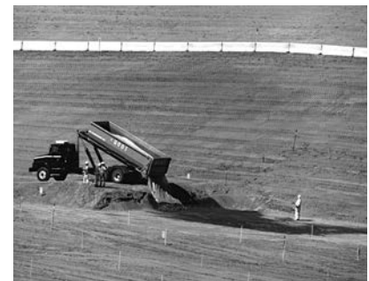
▲ The first load of waste is dumped at Hanford's Environmental Restoration Disposal Facility.
