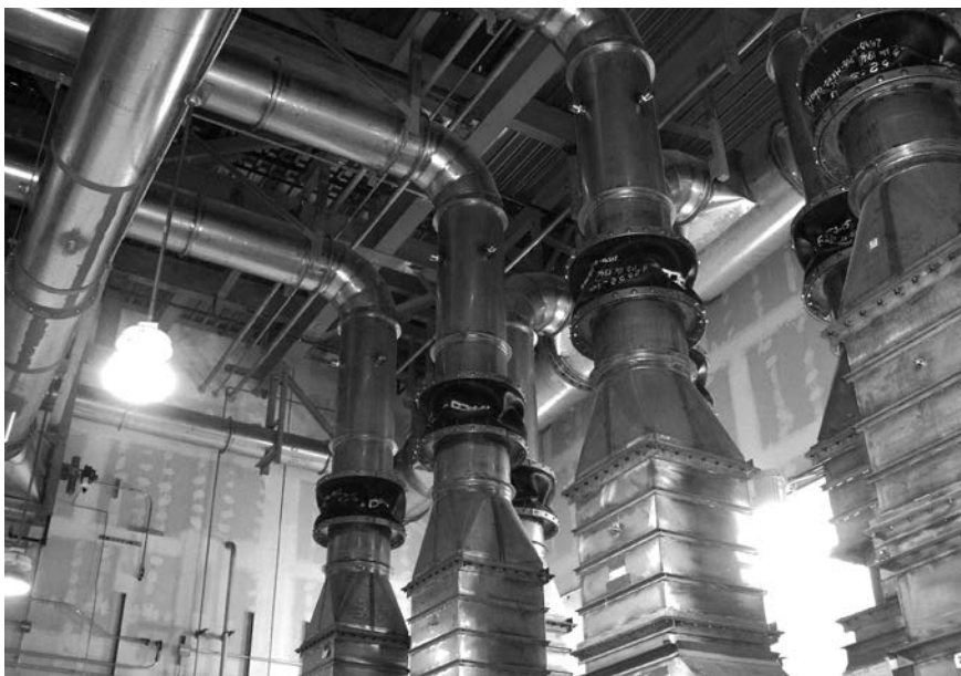
◀ Air handling equipment in the Analytical Laboratory.
