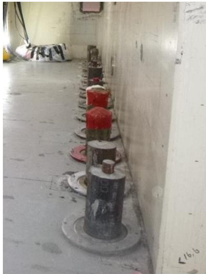
To help support the weight of the hot-cells, the tops of the 13 concrete piles will be attached to the 5' thick B-Cell wall.
