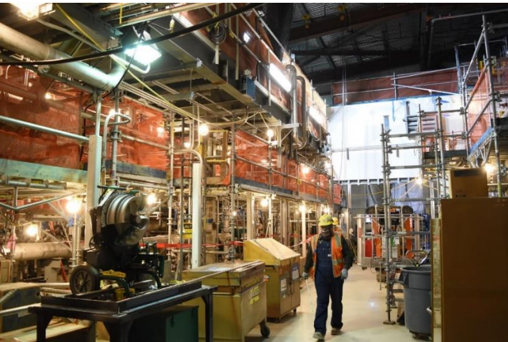
Effluent Management Facility
