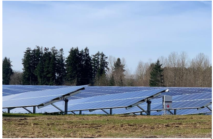
This Keizer-area solar array's capacity is just under 1 MW.
