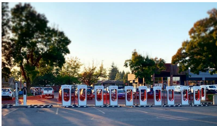
This bank of Tesla chargers was being installed at a northeast Salem shopping center in September 2020.
